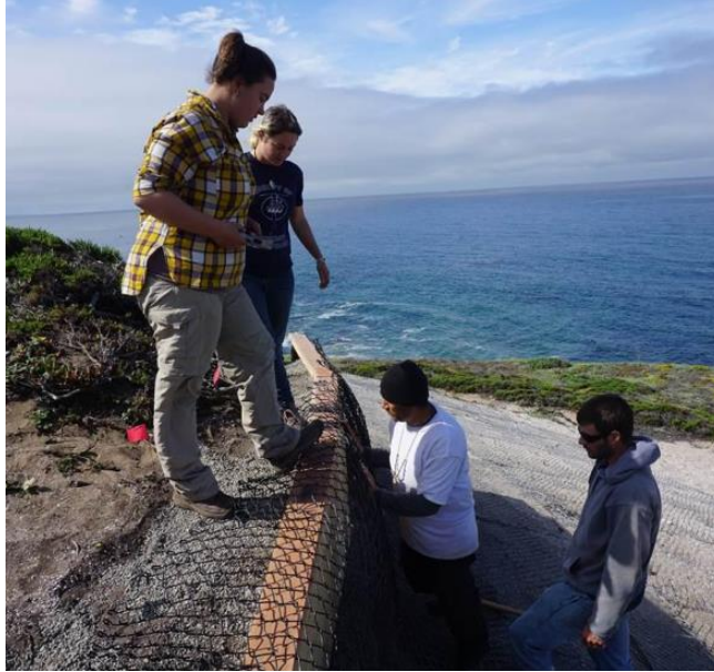
Gabriel Pineida (AMTB) helping to build a retaining wall to protect and preserve archaeological deposits at Sand Hill Bluff with (from left to right) Amanda Dobrov (UCB undergraduate), Michele Maybee (UCB undergraduate), and Rob Cuthrell (UCB archaeologist and AMLT Research Associate).
