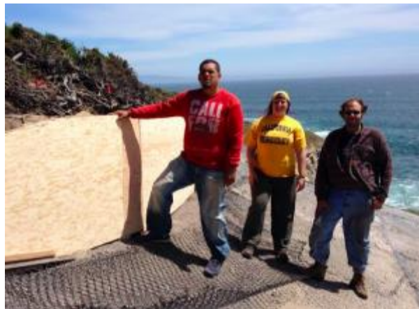
AMTB member Nathan Vasquez (left) works with UCB students Trinity Miller (center) and Charles Woodward (right) to build a retaining wall to stabilize an archaeological site eroding out of a sand dune. Photo by Rob Cuthrell.
